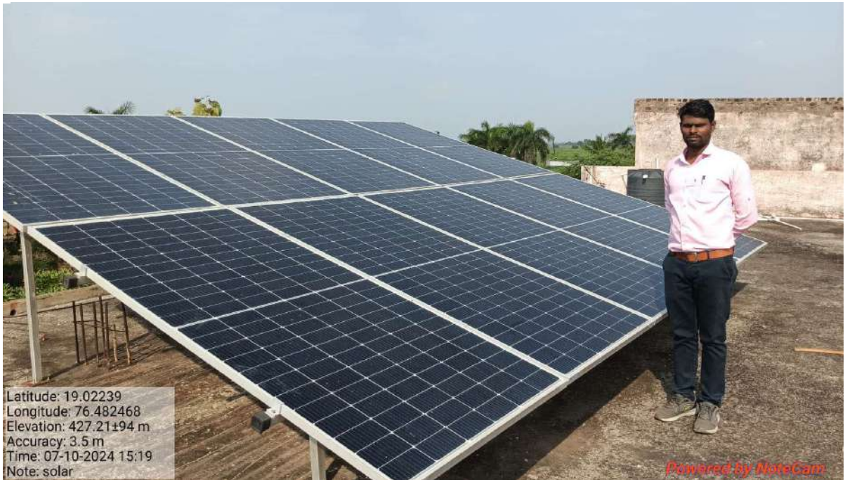
Solar Panels are installed on college roof
