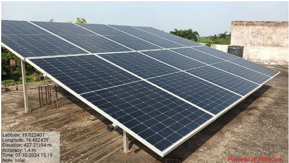
Solar Panels are installed on college roof
